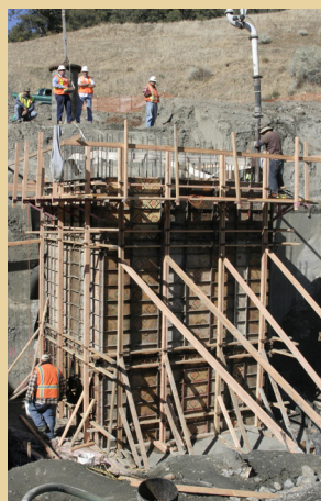
Workers constructing the BEAR TRAP TURNOUT , which provides access to the California Aqueduct—the primary source of water for Tejon Mountain Village.
